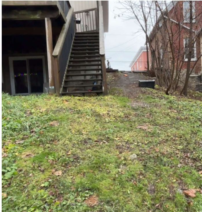
Photograph 1: Upper portion of subject slope in background (east side yard), bottom portion of subject slope in foreground (rear yard). [Looking in project north direction]
